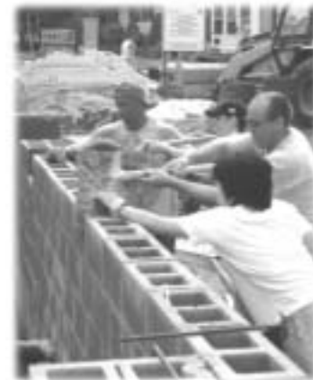
Dedication day is also a workday as these volunteers make progress on the foundation.
