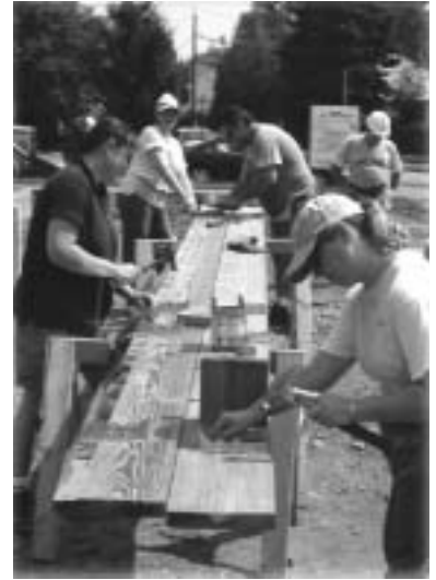
Employees of KMC Telecom work on the Roosevelt Avenue home during one of several company-sponsored workdays.
