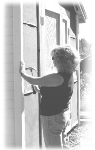
Members of the Clover Hill Reformed Church give their time to the building effort in Lambertville.
