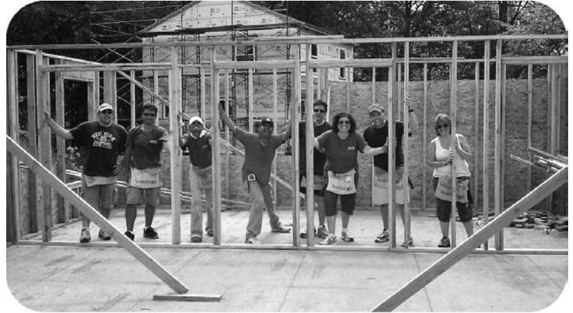
Verizon-Cisco Team members raise a wall of the Harris home in July
