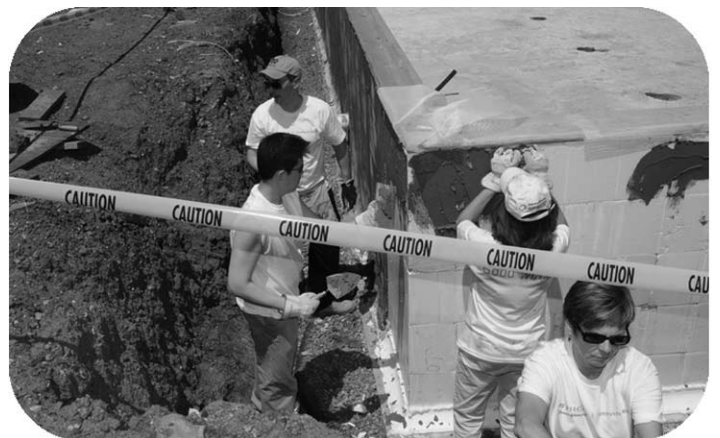
Ethicon employees work on the foundation of 7 Dutch Lane that is sponsored by the Johnson & Johnson family of companies. Team building the Habitat Way!
